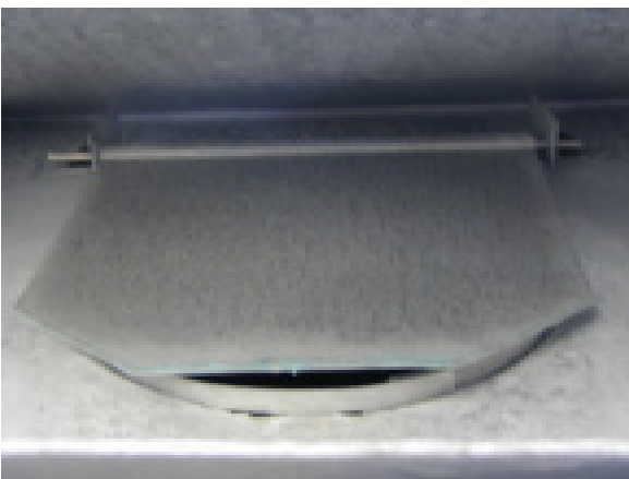
Fig. 11B Improperly closed back draft flapper
